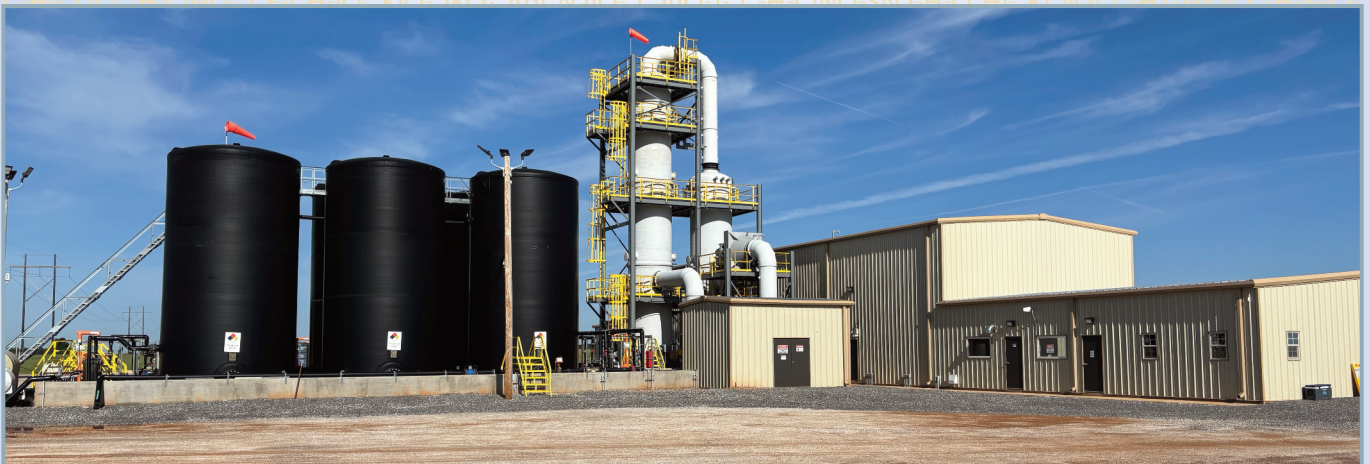
IOsorb ® plant IO#11, Western Oklahoma, USA
